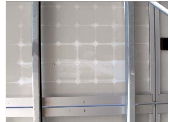
Discoloration of backsheet
