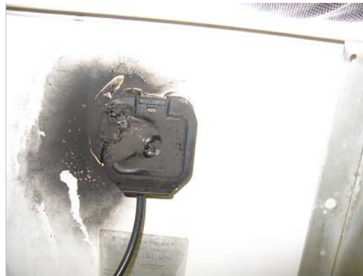
Overheat of connection of output cable
