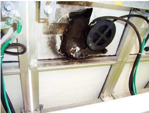
Detachment of junction box
