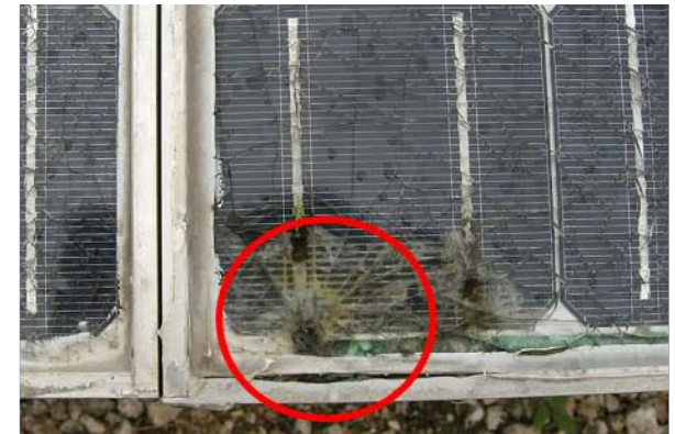
Overheat of connection of busbar
