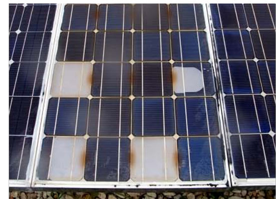
Delamination of encapsulant
