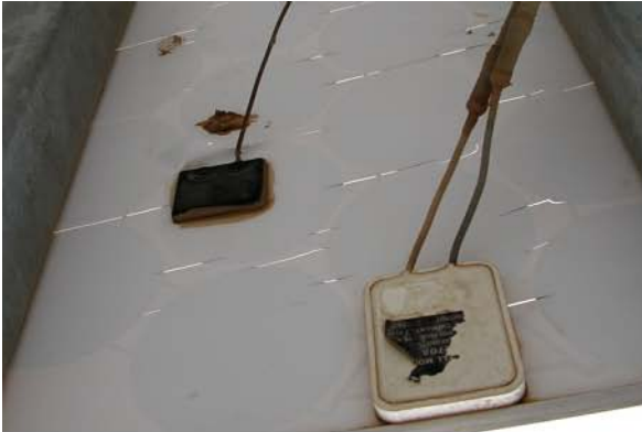
Crack of backsheet
