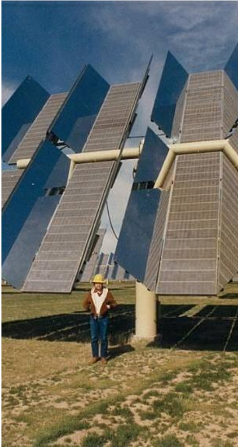
Carissa Plains PV system
